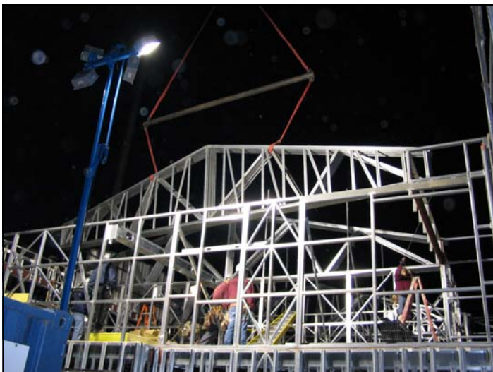
Bay Street in Emeryville: Due to a congested site and the intention to keep the retail stores below open during construction, Daley's set trusses at night. GC: Devcon Construction
